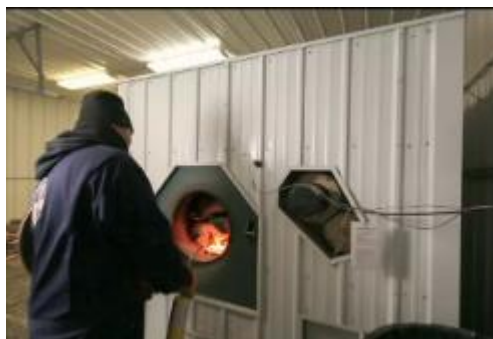
PICTURE 5: GARN BIOMASS BOILER (KOYUKUK, AK)
